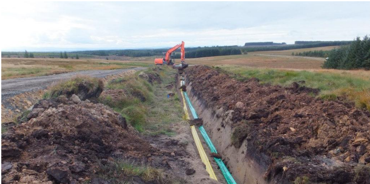
Plate 3: An example photo of a cable being laid using open cut method
