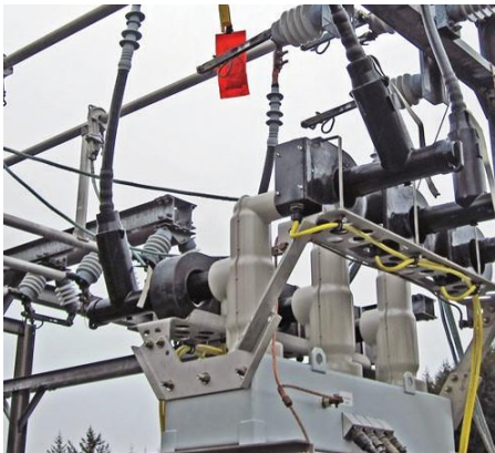
Figure 11: Elbow-Connected G&W Viper Reclosers
